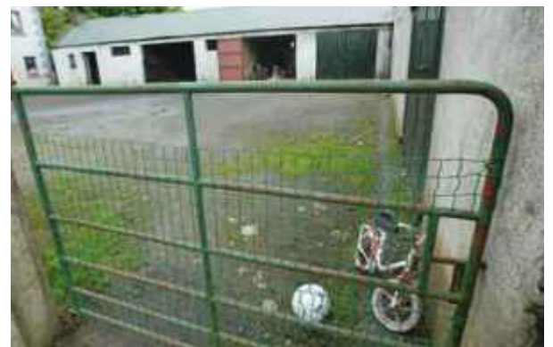
Fence premises and hazardous locations to keep children safe
